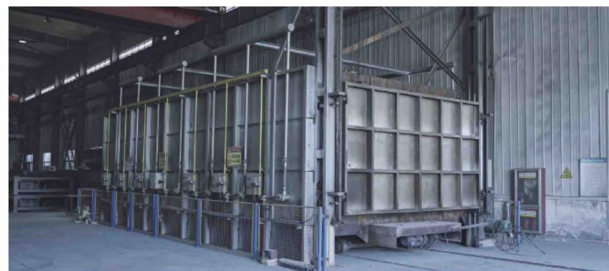
Gas truck style thermal treatment furnace
